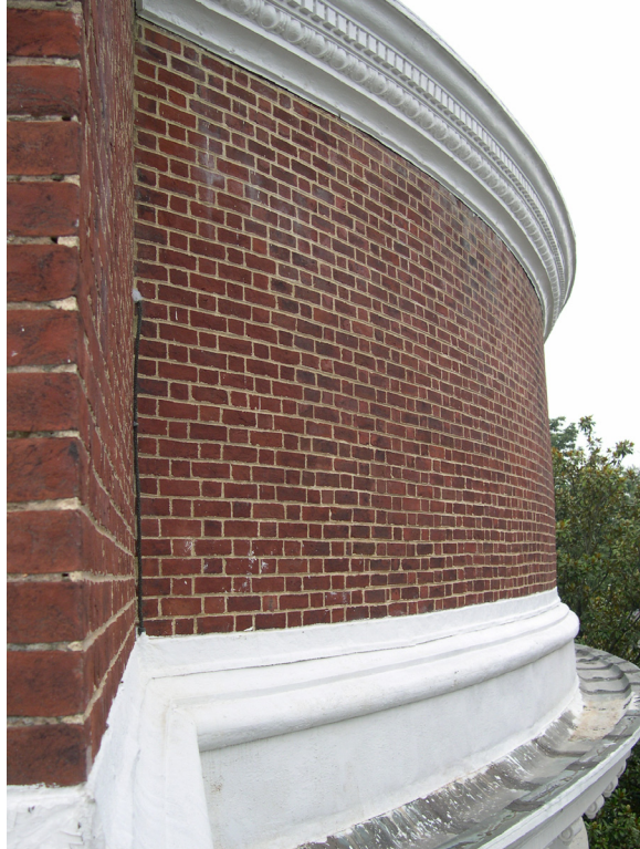
The soffit of the cornice (top), and the attic story (left). [JGWA, 2006]
