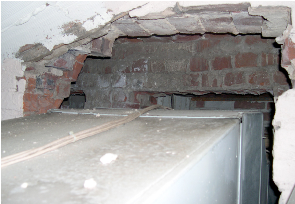
Large duct penetrations have been made in the north wall of the South Portico Attic (402) without providing lintels to support the brick construction above. [JGWA, 2006]
