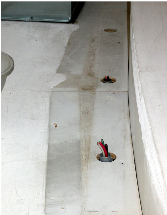
The fluorescent strip lighting fixtures at the base of the dome were removed in December 2006 as part of the mold remediation project. Exposed conductors protruding from conduit remain; these conductors may present an electrical shock hazard. [JGWA, 2006 (top), 2007 (bottom)]
