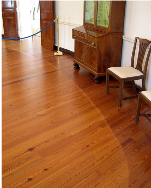
The floor finish in the President's Reception Room (Upper West Oval Room 201) is discolored as a result of UV degradation. This was made apparent by the removal of the large oval rug that was located in the center of the room. [JGWA, 2006]
