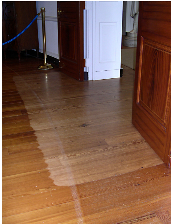
Floor sanding in the Center Hall (C202/C203) was continued through the east entry of the President's Reception Room (Upper West Oval Room 201). This refinishing work and the perimeter abrasion from a large oval rug have caused discoloration and uneven wear in the heart pine flooring. [JGWA, 2006]
