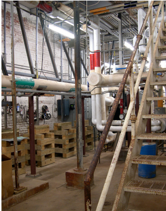
Generations of temporary shoring have been introduced in the Mechanical Room beneath the north portico to support the ceiling and terrace construction above. [JGWA, 2006]
