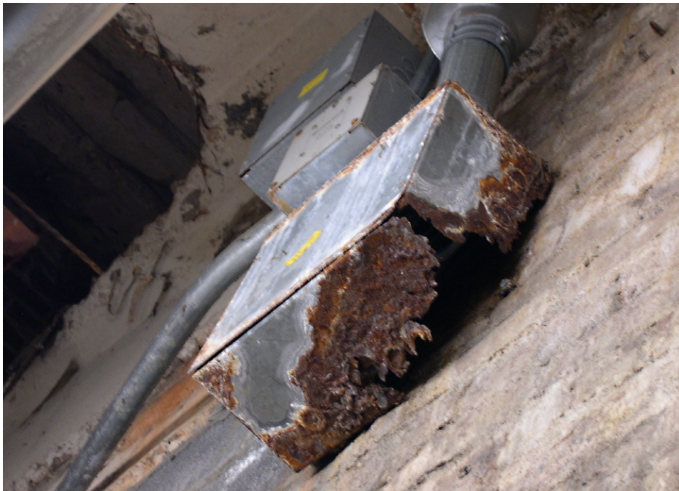
Significant problems with water infiltration in the Mechanical Room beneath the north portico have lead to advanced deterioration of equipment and fixtures. [JGWA, 2006]
