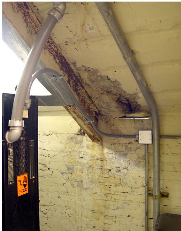
The exposed steel beam supporting the sloped concrete ceiling of Elevator Machine Room (110A) has significant surface rust. The rust is more advanced at the beam's bearing point in the north wall. Galvanized sheet metal and acrylic glazing have been installed above the elevator machinery to protect the equipment from water infiltration occurring in the north portico steps above. [JGWA, 2006]
