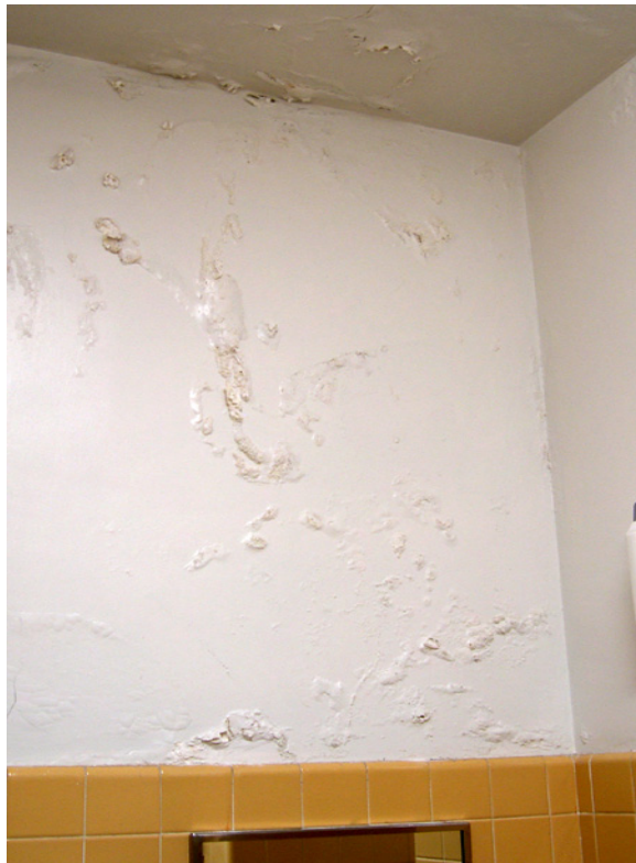
The plaster wall and ceiling surfaces in the northeast corner of the Men's Toilet Room (T113) are badly blistered. The plaster is friable, and the painted finish is peeling as a result of water infiltration. [JGWA, 2006]
