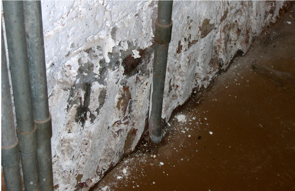
There is rising damp in the masonry construction of the north and east walls of Mechanical Room (108). The painted wall finish is peeling, and efflorescence has formed on the masonry. [JGWA, 2006]
