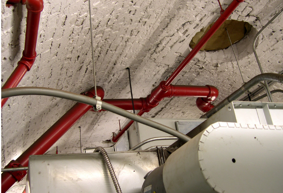
The clearance space for mechanical, electrical, telephone, and sprinkler equipment in Mechanical Room (108) is inadequate and does not meet current building codes. [JGWA, 2006]
