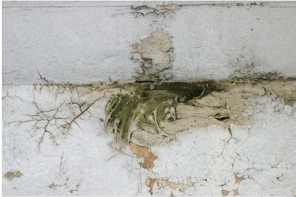
Rotunda, Roof. Inadequate attempts have been made to cover areas of exposed sheet metal on the steps at the base of the dome with smeared sealant. The sealant is supporting the growth of algae.[JGWA, 2006]
