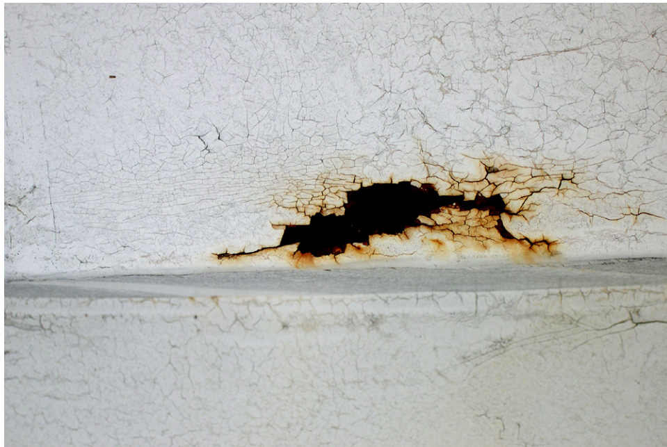
Rotunda, Roof. The painted finish on the terne-coated roofing of the dome is crazed and peeling; the underlying sheet metal is rusting through. [JGWA, 2006]
