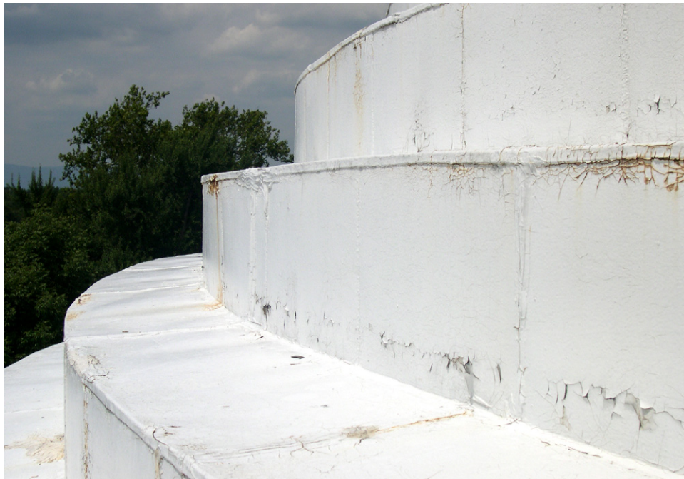
Rotunda, Roof. The painted finish on the terne-coated sheet metal roofing of the dome is crazed and rust stained; this condition is pronounced on the north elevation. [JGWA, 2006]
