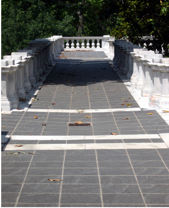
West Terrace. Debris from the magnolia trees accumulates on the terrace. [JGWA, 2006]
