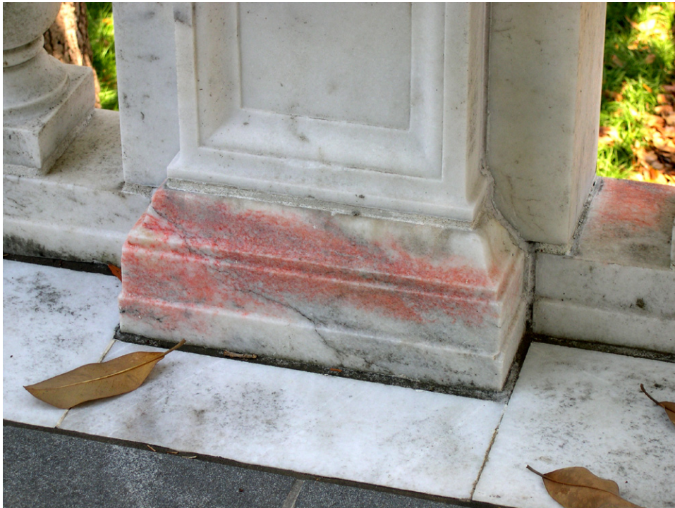
West Terrace. There is vivid orange “staining” along the bottom rails of the marble balustrades; this appears to be subsurface biological growth. [JGWA, 2006]
