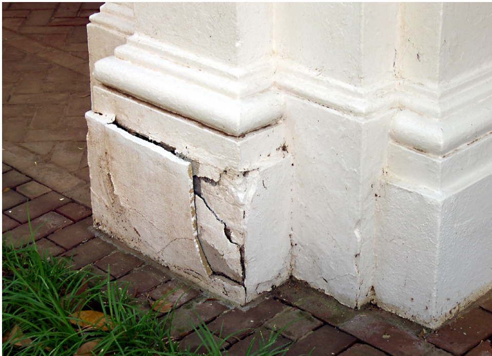
East Colonnade, West Elevation. The parging on the pier at the north end of the colonnade has separated from the underlying brick construction. [JGWA, 2006]
