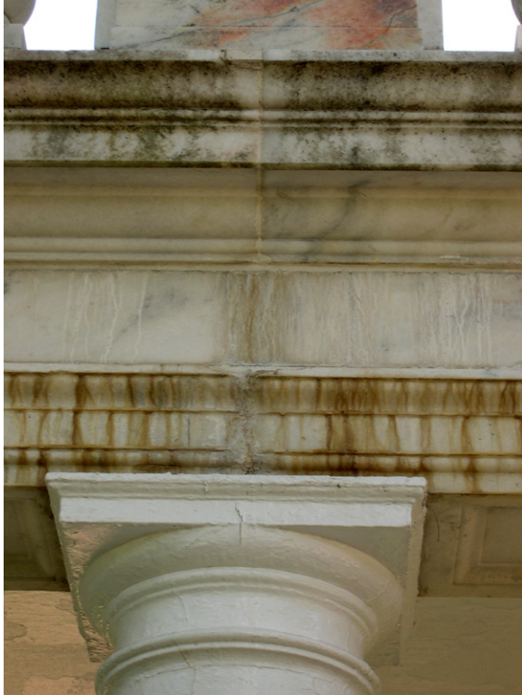
West Colonnade, West Elevation. There are lime-run (calcium carbonate) deposits at the vertical joints in the marble entablature, and rust colored staining on the architrave. This deterioration has resulted from water percolating through the terrace construction above. [JGWA, 2006]
