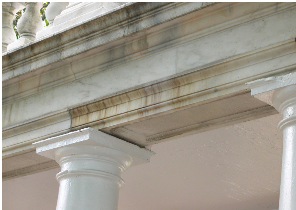
East Colonnade, East Elevation. The marble entablature and soffit have been soiled and stained by rainwater run-off, originating in the terrace construction above. [JGWA, 2006]
