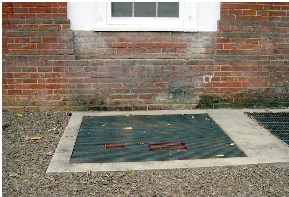
Northeast Wing, North Elevation. The painted surfaces have chalked and stained the brickwork. There is dark biological staining on the brick near the rusted areaway grates. [JGWA, 2006]
