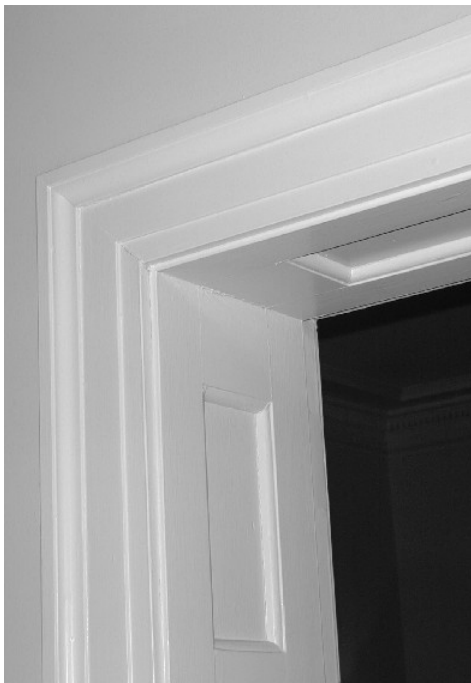
jamb of the first-story main room when the pocket door was removed (left).
