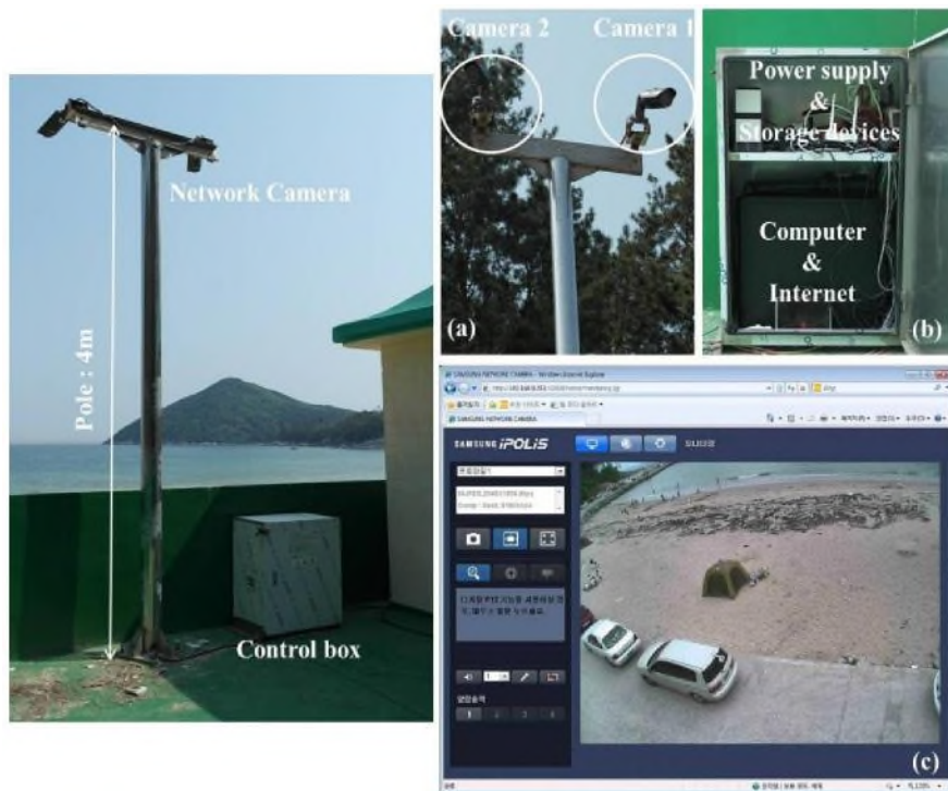
Fig. 2. The structure of the network camera system: (a) a network camera setting on a 4-m-high pole (SNO-7080R), (b) the structure of the control box, and (c) the web browser for real-time monitoring.
